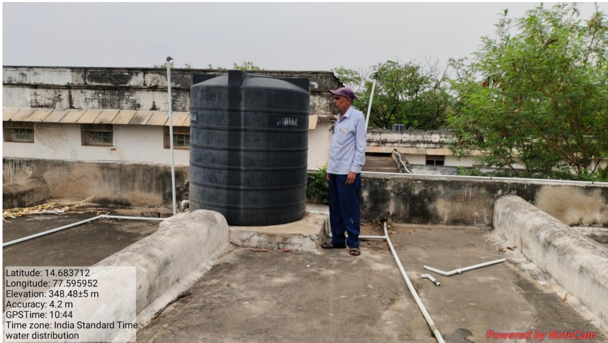
Main tank supplies water to Library, Ladies waiting room, Microbiology
