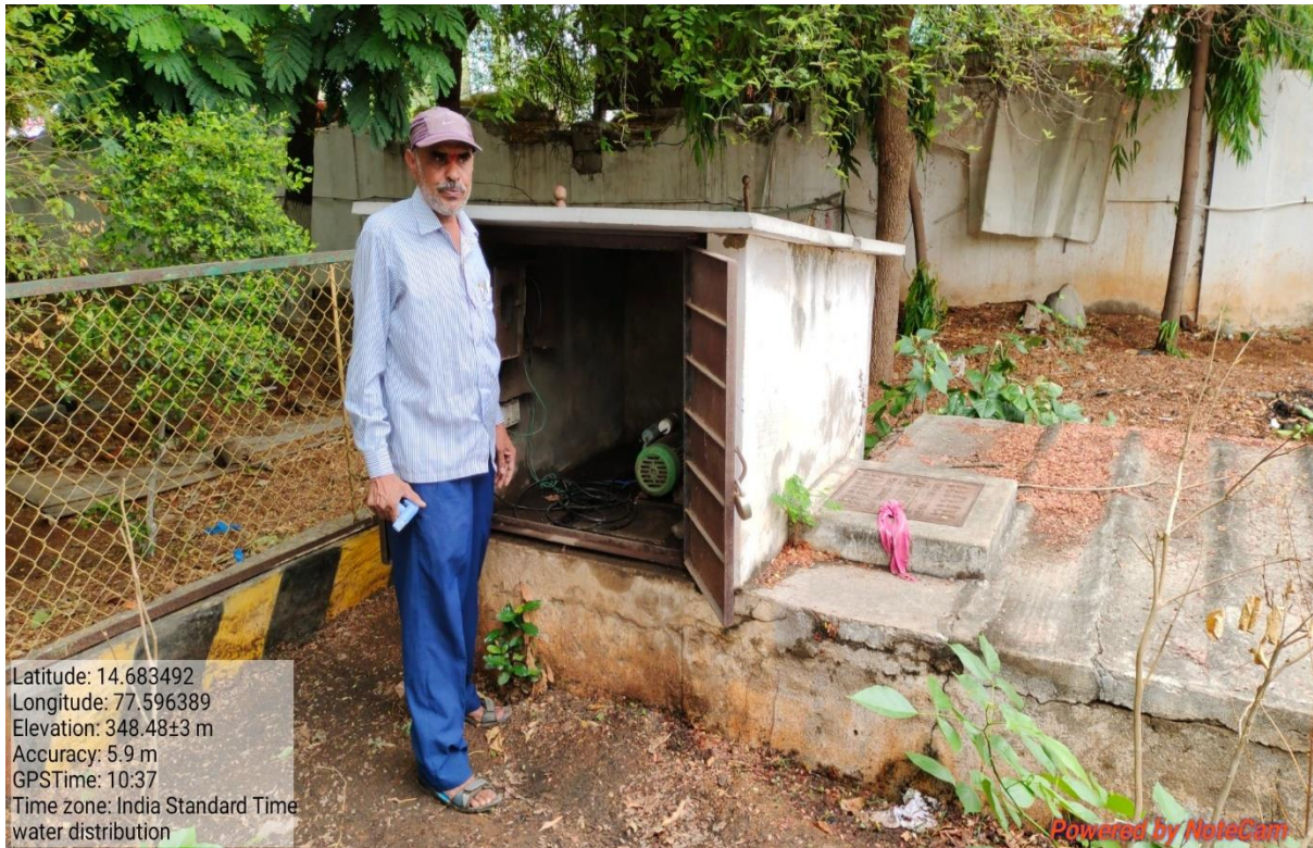
Mr. Ranga, In-Charge of water maintenance in the college. Main Water pump.
