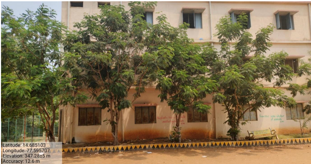
Luxuriant growth of plants with rain water from the terrace in the Commerce block
