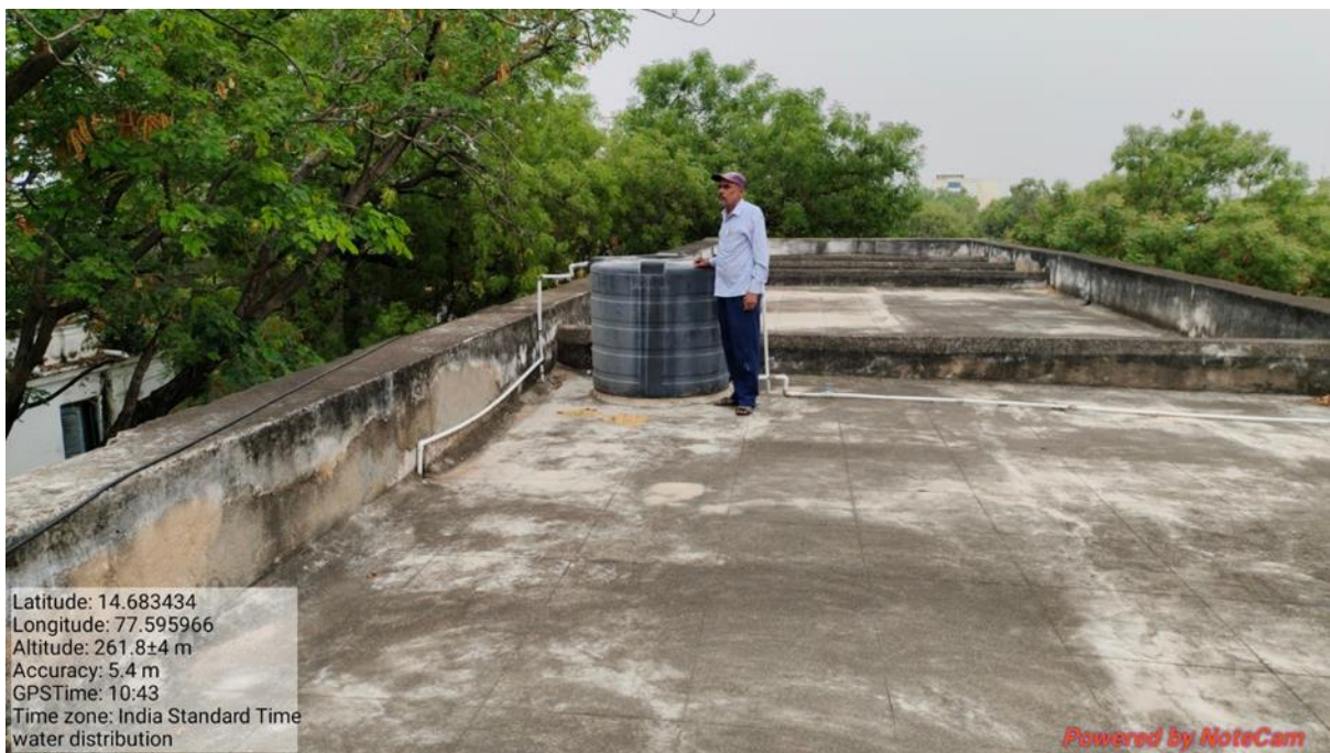
Water tank Supplies water to the Principal Chamber and Office Room.
