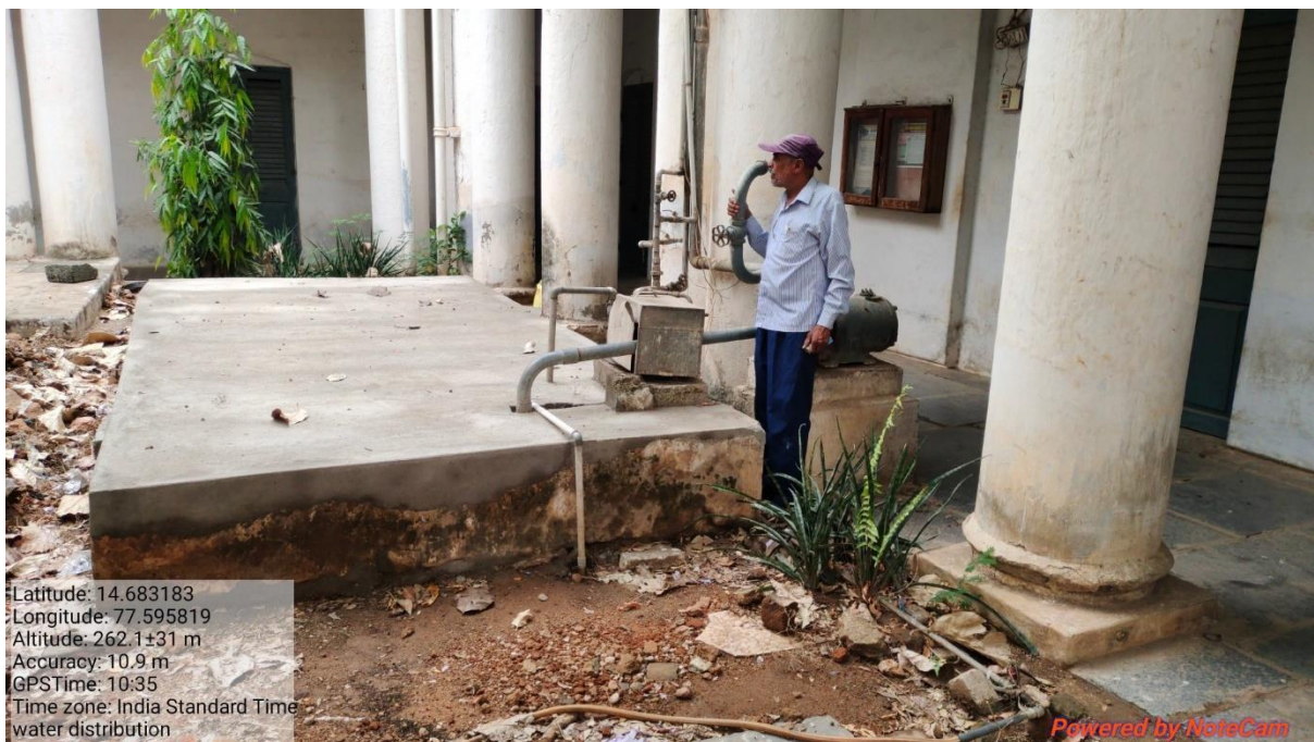
Tap water Sump at Physics Department from which water is distributed to Physics, Chemistry, Biotechnology and Examination sections.
